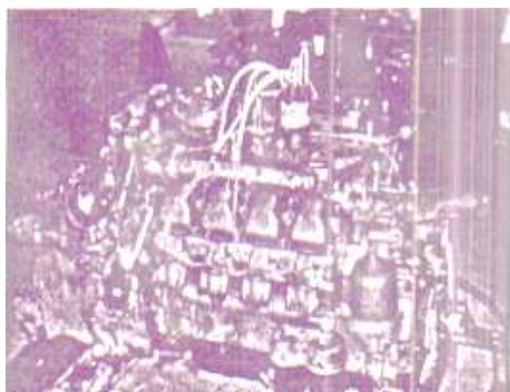
Fig. 1. Overall view of a naturally aspirated gas engine with transistorized ignition systems
