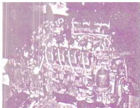
Fig. 2. Overall view of a naturally aspirated gas engine with microprocessor ignition and control systems
